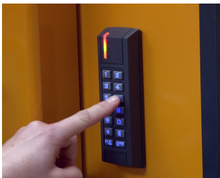
A digital auto lock enables baler loading but restricts access to run a press cycle.
